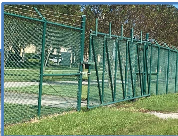
Photo 4-7 Perimeter fence gate space greater than 6 inches
