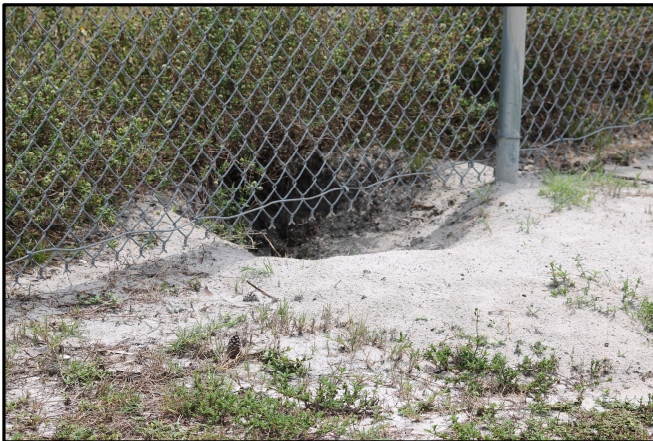
Photo 3. Breach in perimeter fence at PMP.
