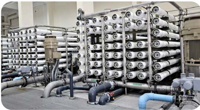
Membrane Filtration for Water Treatment
